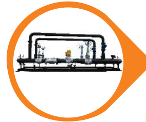
Pressure Reducing & Desuper Heating System
